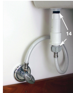
14. Check for leaks around threaded connections (If leak is present, see "Corrective steps for leaks"). 15. Flush toilet. Replace lid.
